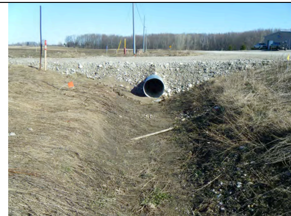
PLATE 4 NEW DRAINAGE UNDER NEW GRAVEL ENTRANCE
