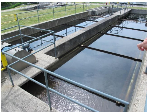
Final Settling Tanks
