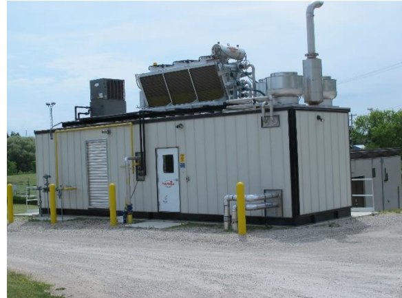
Gasification Generator – this unit converts methane gas to electrical energy that is then available for use by the plant; any excess energy is then fed into the electricity grid. This “offsetting” accounts for the reduced electricity consumption that is shown in the years 2014-15 (See Figure 5)
